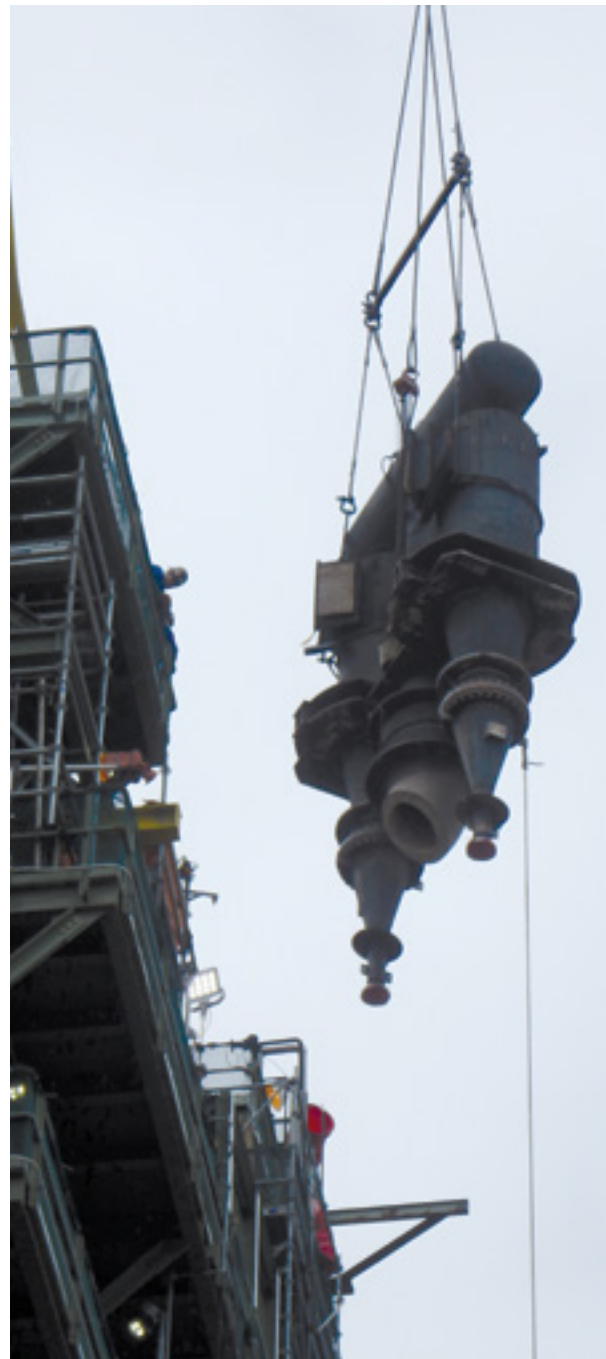
During this turnaround, thousands of pounds of equipment (both new and old) were added and removed from the FCC structure, such as the removal of some old cyclones shown here. Each of these crane lifts required detailed planning to ensure that they were completed safely.
